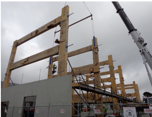
Merrit Building, Christchurch, New Zealand (courtesy of Andy Buchanan)
